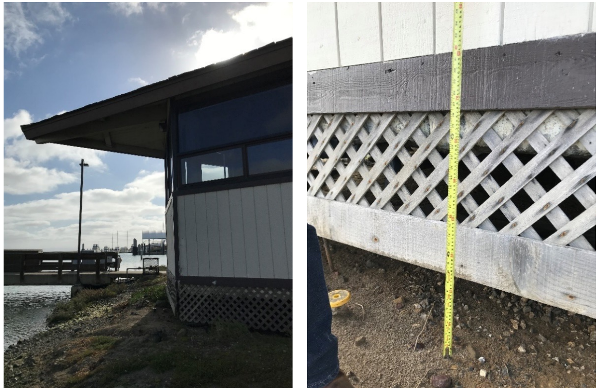
Figure 22. Oyster Point Marina – Harbormaster Building Undermined Foundation (with skirt)
