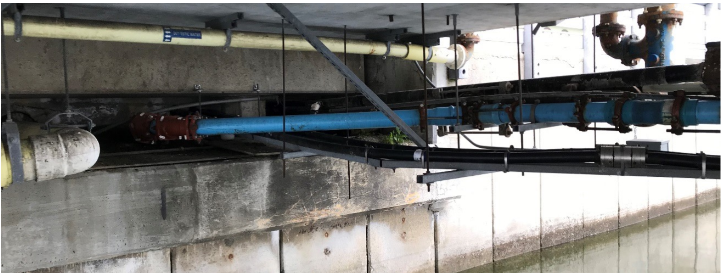
Figure 13. Johnson Pier, Under-deck Utilities at Bulkhead
