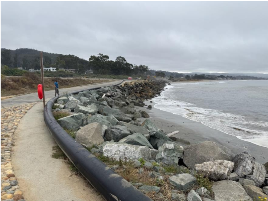
Pumping sand to north end began on August 28, 2025. A total of 10,000 cy was placed.
